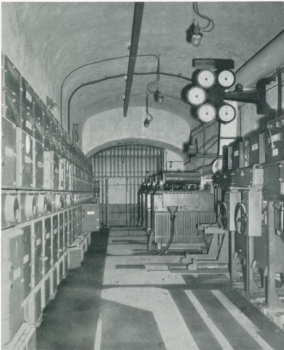
A power plant in the Maginot Line. Systems like this kept living conditions in the fortifications pleasant, with air conditioning, electric kitchens and moving pictures.
