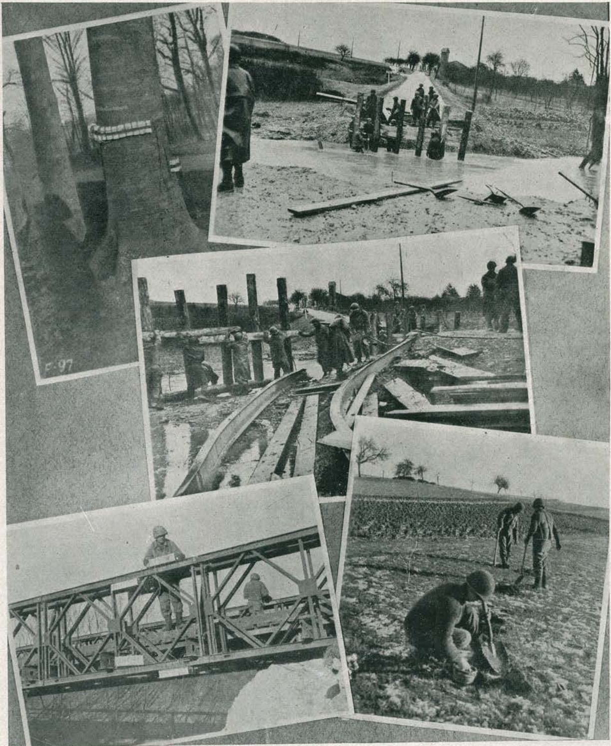
Before our withdrawal to the "Bulge" sector road blocks are erected and fields are mined.
